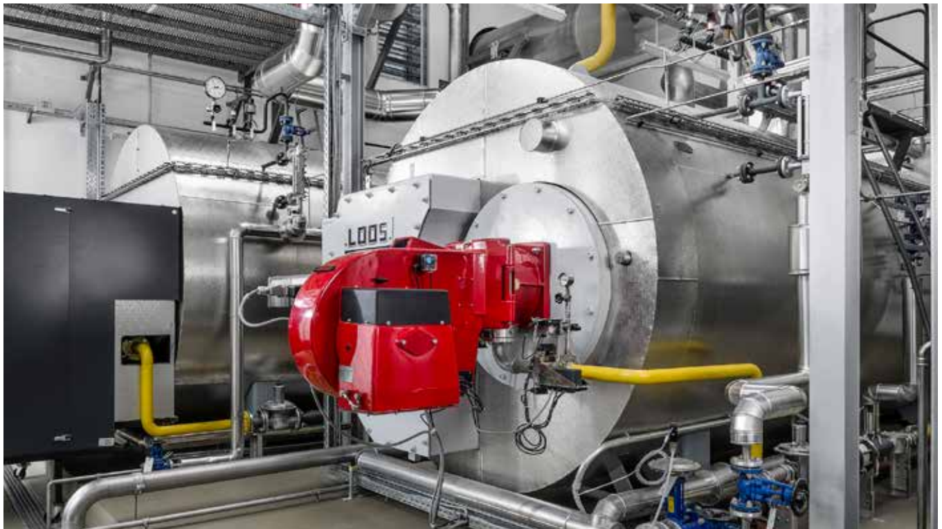
The modernised steam boilers with oxygen- and speed-controlled natural gas burners at Oettinger Brewery.
