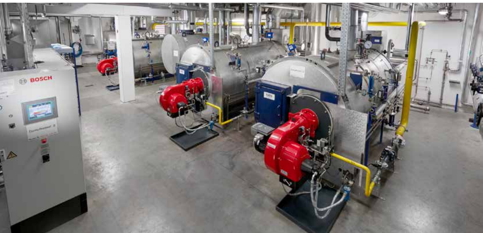
Sutter's process heat supply works with greater efficiency after the successful modernisation.
