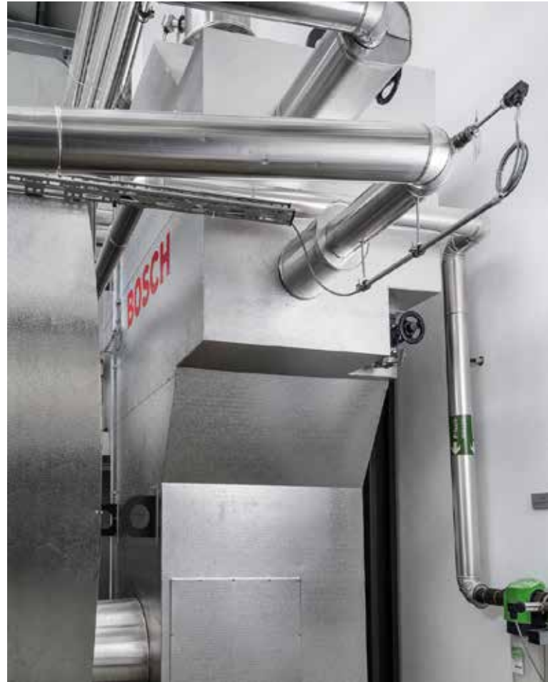
Using waste heat for preheating feed water saves fuel and protects the environment.
