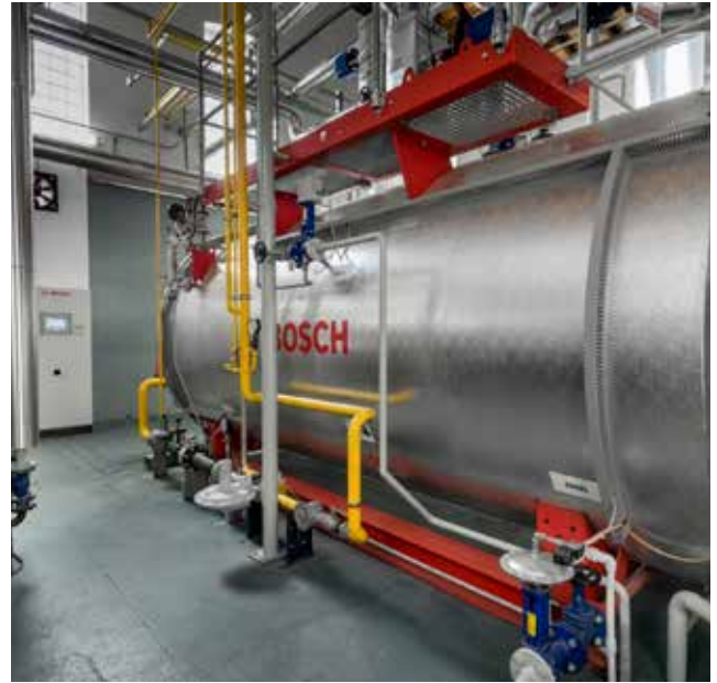
The times when it was necessary to have a constant presence in the boiler house have long since gone.
